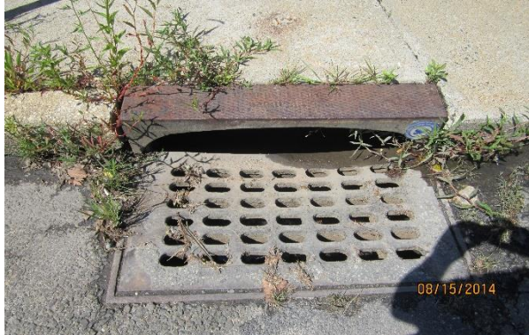
Storm Drain Inlets
